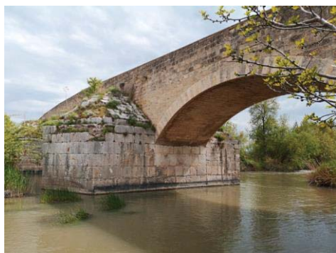
Fig. 2. Canosa. View of the western pier of the bridge. (photo by G. Germanò)
