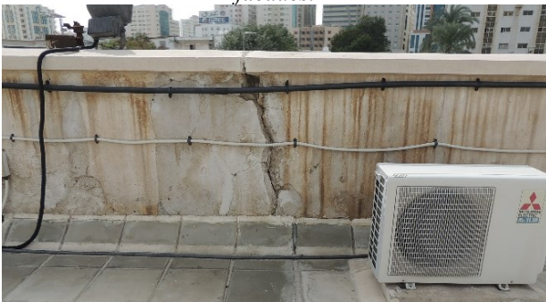
Fig. 4. Material deterioration of the museum structure as shown on the rooftop.
