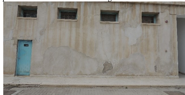
Fig. 2. Material loss in one of the museum's internal facades.
