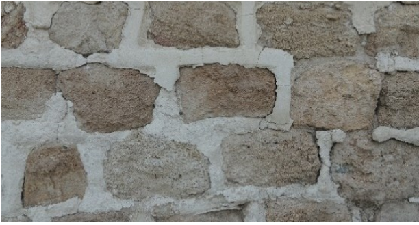
Fig. 3. Material loss in one of the museum's external facades.
