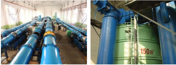
(a) DN500 ~ DN1600 large water flow standard facility (NWLFMS)
