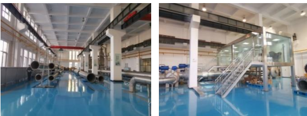
(b) DN800 large water flow standard facility(HBIM)
